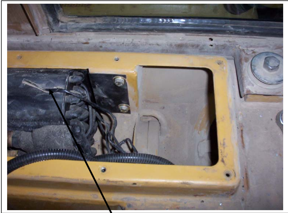
Thermostat probe location
